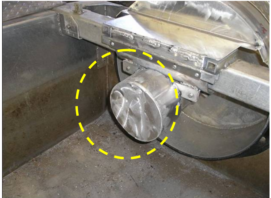
The shaft must be completely encapsulated with no moving parts exposed.
