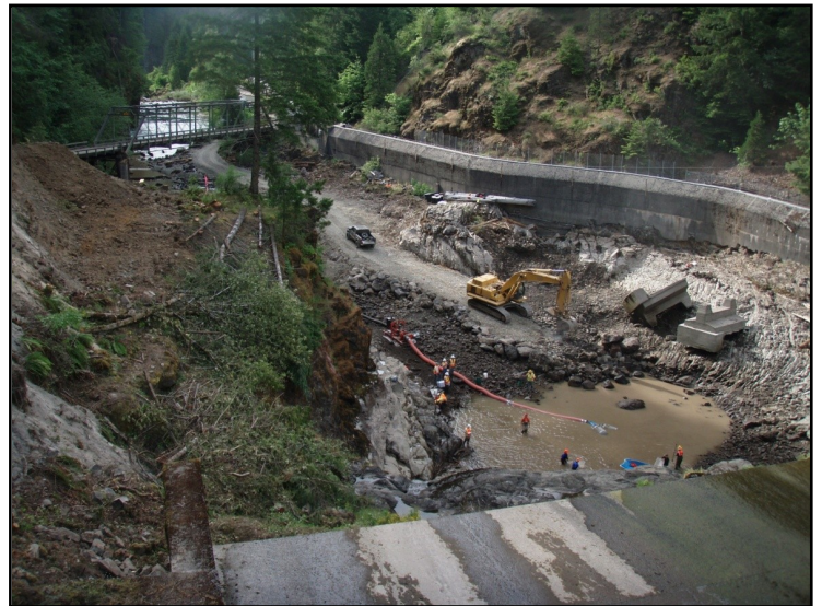
Residual pool near end of day three, fish salvage and pumping in progress as excavator pioneers access for pump (note fish screen on pump intake). Photo: P. Sighting
