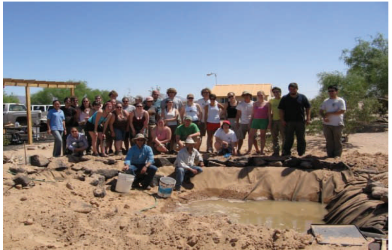
Oregon State University Fisheries and Wildlife Club assisting with the construction of artificial ponds for endangered desert pupfish ( Cyprinodon macularis ) at the El Pinacate Biosphere Reserve—Puerto Penasco.
